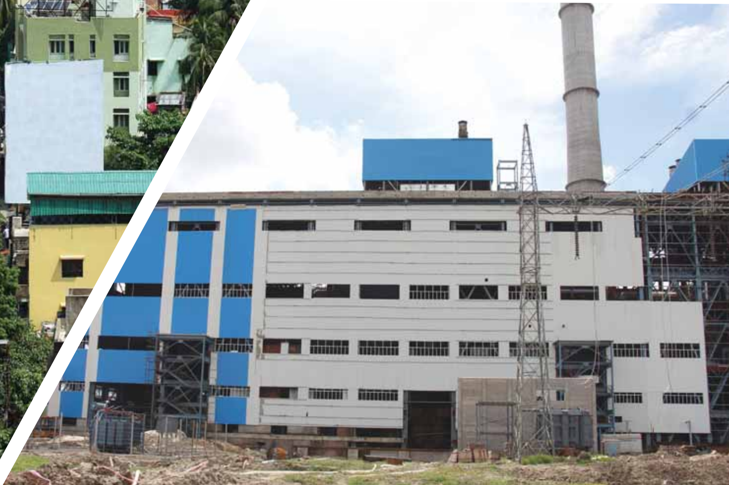
Construction of 3 X 150 MW Thermal Power Project for IPC(H)L, Haldia in progress
