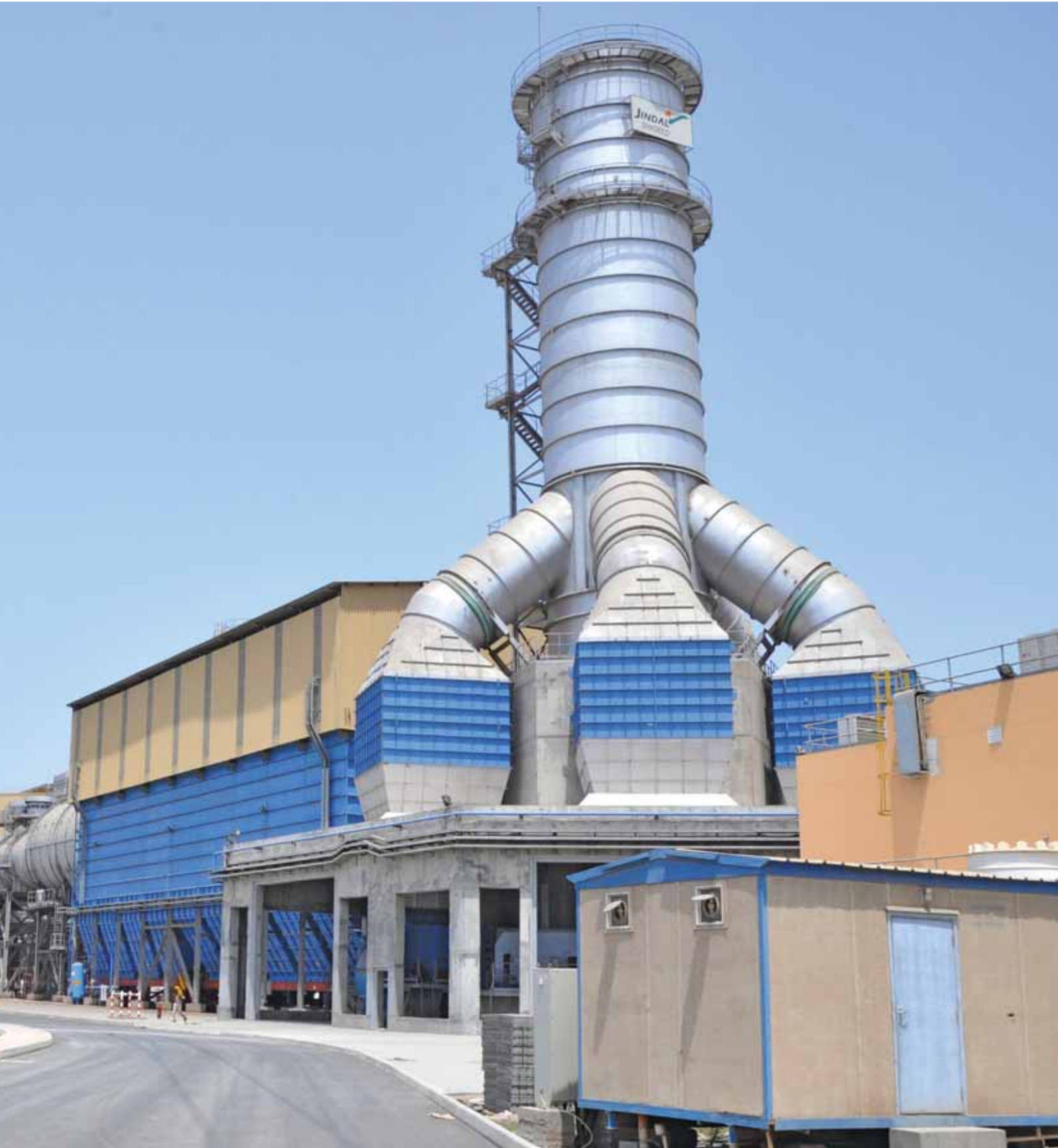
Cement Plant – UMM – BAB Doha, Qatar
