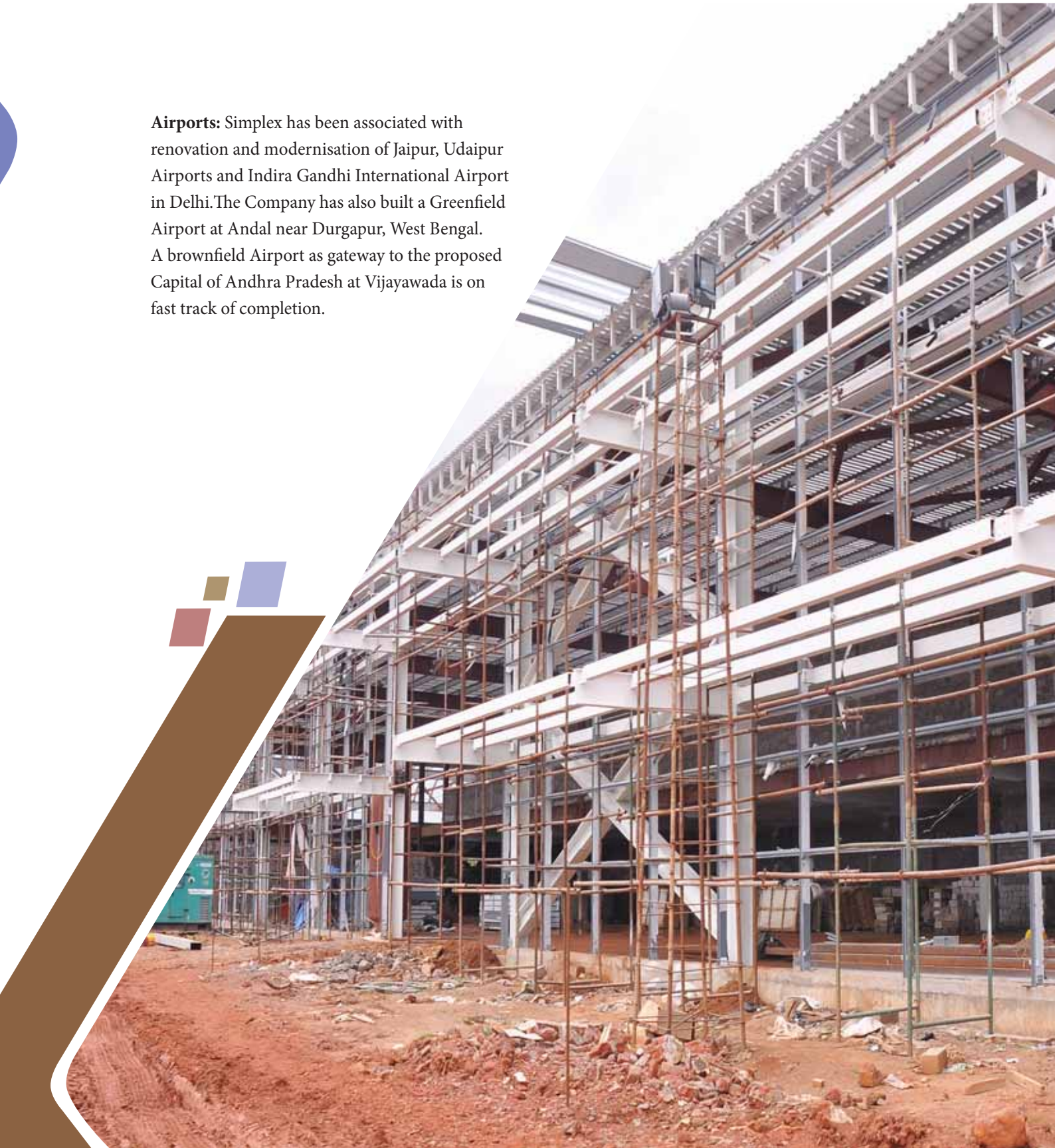
DGU Facade Frame over Structural Work for new Vijayawada Airport Terminal, Andhra Pradesh
