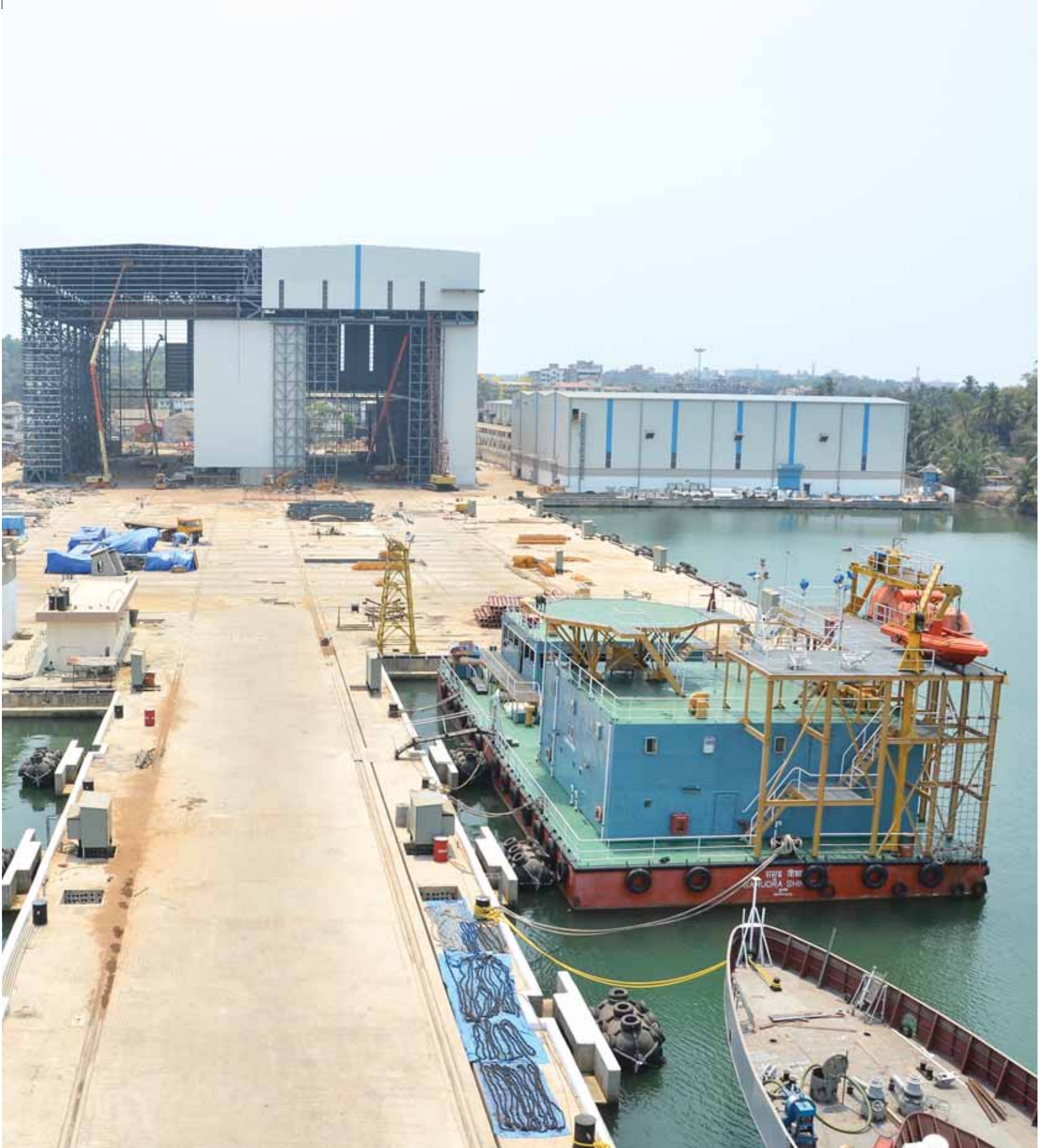
Modernisation of Goa Shipyard Limited (Phase 3A works) under advanced stage of completion at Vasco-da-Gama, Goa
