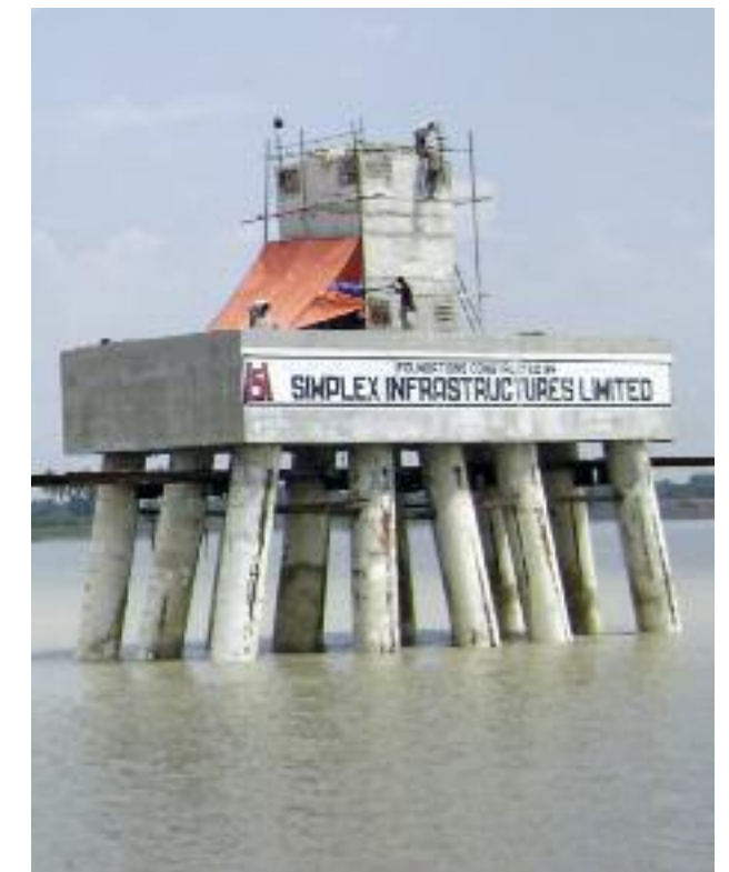
Raked Steel Pile & Cap Foundation for 240M High Transmission Tower for 400KV DC Line across Hooghly River at Raichak to evacuate Power from CESC’s Haldia unit to Kolkata
