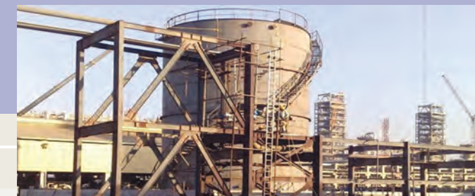
View of bulk chemical storage tank for Reliance Petrochem Ltd at Jamnagar, Gujarat.
